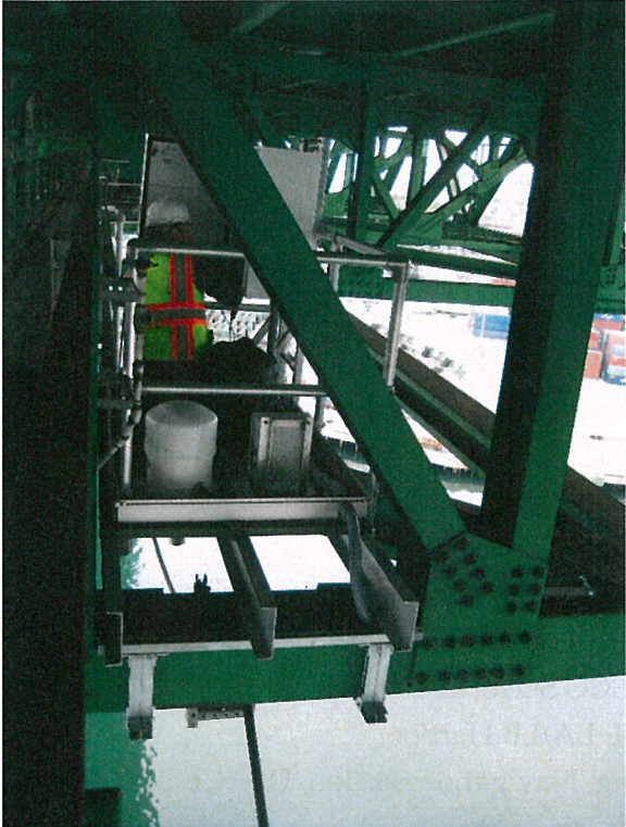
Images 1 and 2. Air Gap Sensor Installation on the Vincent Thomas Bridge.
