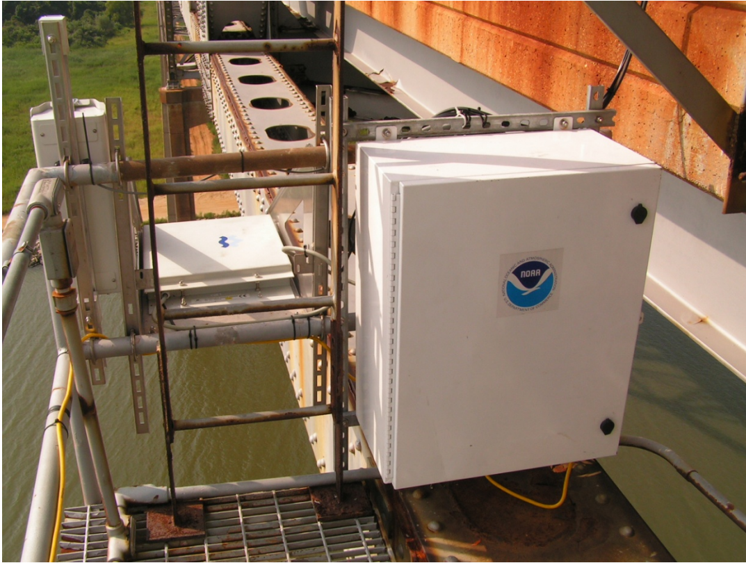
Figure 3-2. Side view of Reedy Point Bridge Miros mount.
